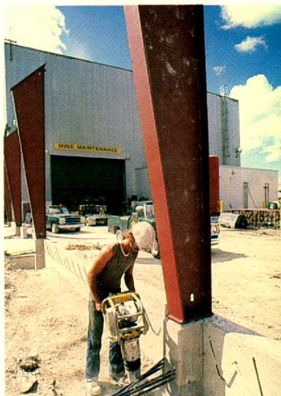
Steel being erected for expansion of Lornex mine maintenance building. The addition will enable the facility to handle the expanded array of trucks, shovels and other equipment.
