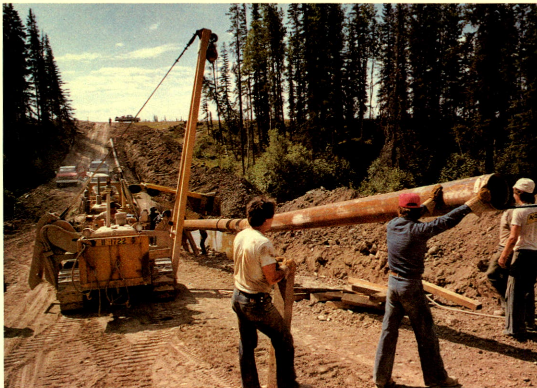
This gas pipeline project in northwestern British Columbia undertaken by Pacific Northern Pipeline Ltd. was partially financed by London Life as part of its $90 million private placement program during 1982. London Life has more than $4.4 billion invested in real estate, bonds, mortgages, stocks and other assets.
