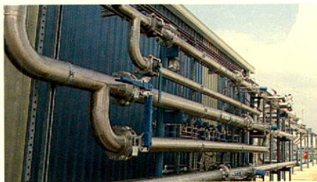
Ultra High Purity Piping
