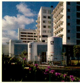
Medical Oxygen Installation
