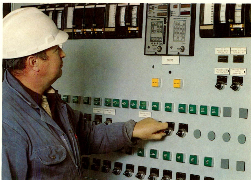
Vane Orcutt monitoring the master control panel of the water plant at West Eagle Unit No. 1.
