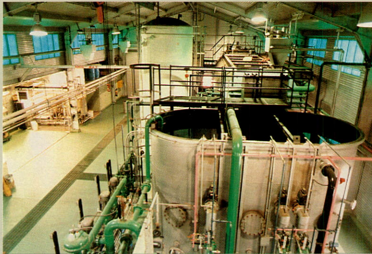
The freshwater treatment plant at West Eagle Unit No. 1
