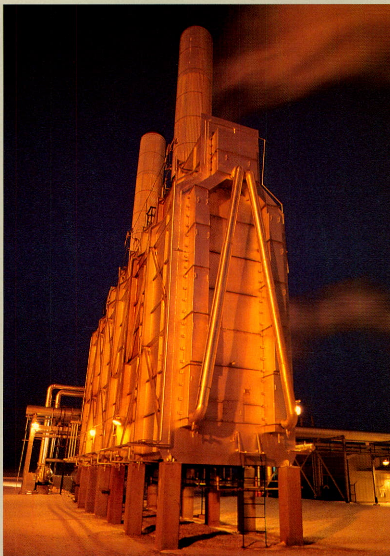
Part of the facilities at the Carstairs Natural Gas processing plant north of Calgary
