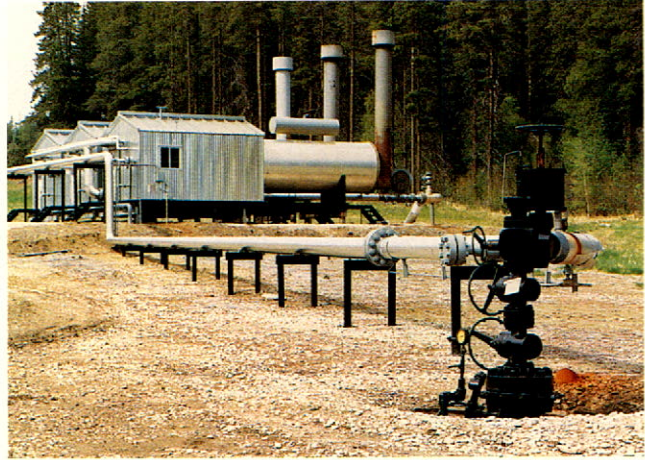
A producing well in the South Wapiti natural gas field.
