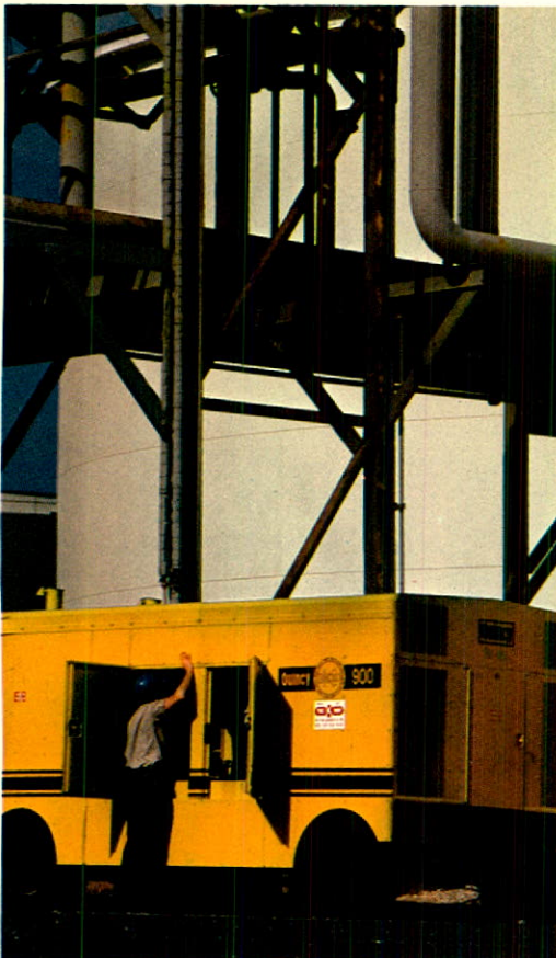
Above: Service representative conducts maintenance inspection of a Quincy helical screw compressor which provides compressed air for pneumatic power vital to operations at a major Gulf Coast oil refinery.
