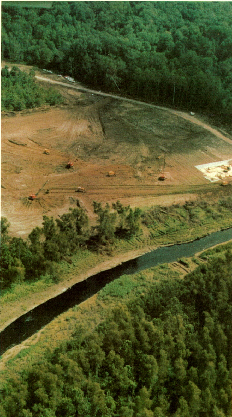
Supreme Contractors, Inc., acquired in mid-1980, prepares access roads and drilling sites in southern Louisiana
