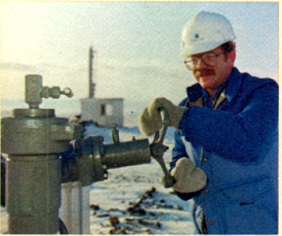
Top: Construction of a new gas compressor station at Heart River began in late 1982.
