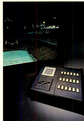
GE's 1000 watts Multi-Vapour® high intensity discharge lamps and remote control wiring system in use at Copps Coliseum, Hamilton, Ontario.
