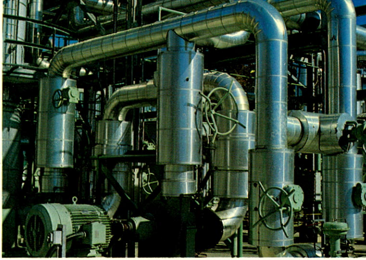
Unique new West Virginia plant separates natural gas and carbon dioxide, allowing useful recovery of both gases.
