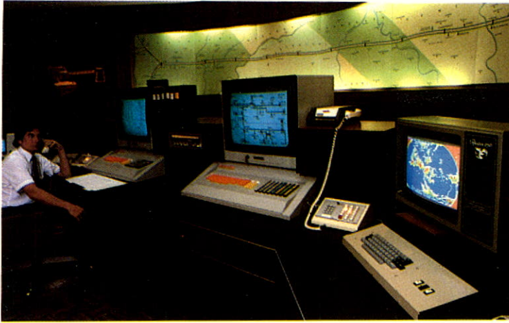
Gas production flow through Columbia's Louisiana-West Virginia pipeline is monitored from central control room in Houston, Texas.
