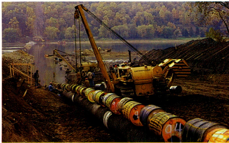
Columbia's capacity to transmit gas was increased by this 1981 project to install a larger pipeline across the Susquehanna River in Pennsylvania. Barrels support the pipe while it is pulled across, before lowering into river bottom trench.
