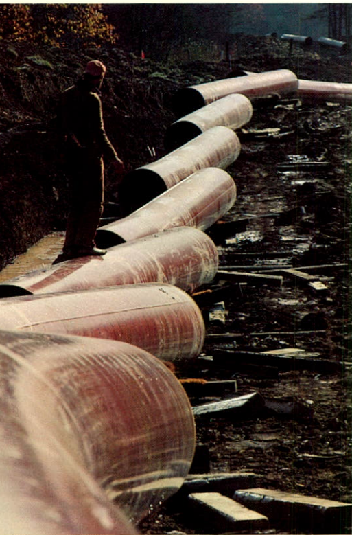
Pipeline sections 30 inches in diameter await the construction crew on a West Virginia expansion project.
