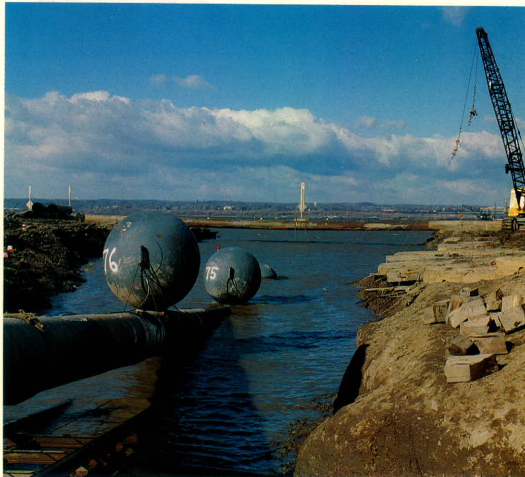
A 7,000-foot crossing of the Delaware River south of Philadelphia extended Columbia's transmission lines into New Jersey in 1987. The line was pulled across as sections were welded together. Buoys were released to let the line settle into a trench.
