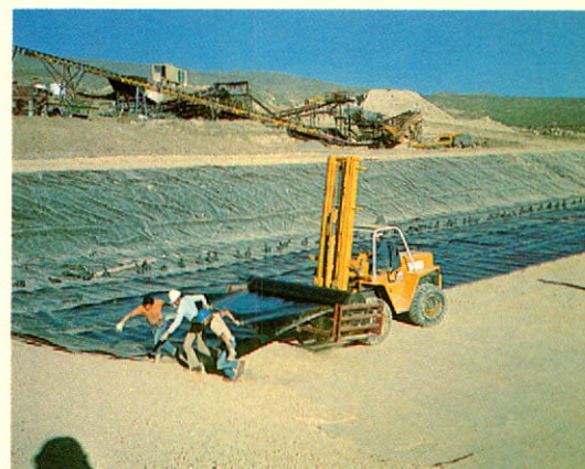
Carlin, Nevada: heap-leaching ponds under \Delta construction at the new Buckhorn operation.
