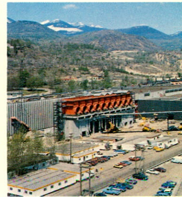
The new zinc electrolytic and melting plant at Trail, the world's largest, is setting the standard for electrolytic zinc technology.
