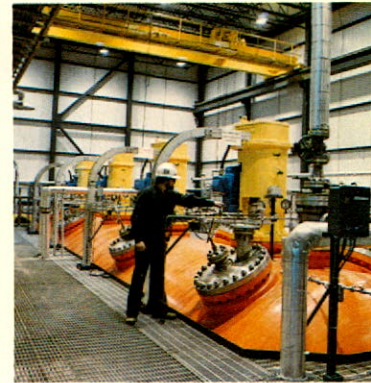
The autoclave in the new zinc pressure leaching plant, an innovation that has resulted in more efficiency and a cleaner working environment.
