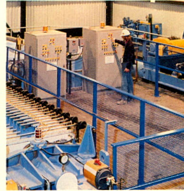
The two Lasta filter presses are on the top floor of the solids separation plant of the zinc fume leach project at Trail.
