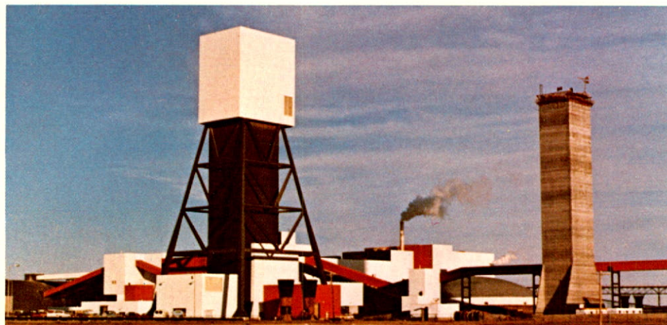
New slipformed concrete headframe will join existing counterpart to increase production at Vade, Saskatchewan potash operations to 1.2 million tons a year.
