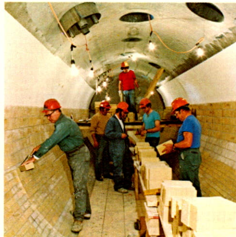
Workmen at Trail line autoclave pressure vessel, an integral part of the new pressure leaching process.
