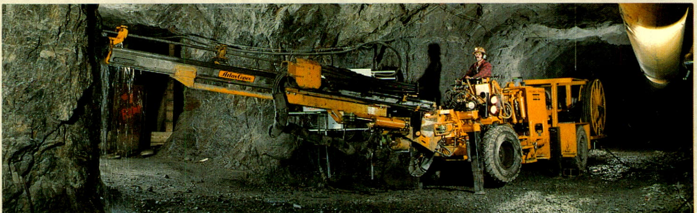
A rubber tired jumbo drill with three 20-foot booms is part of the mechanization mining program at the Sullivan mine.
