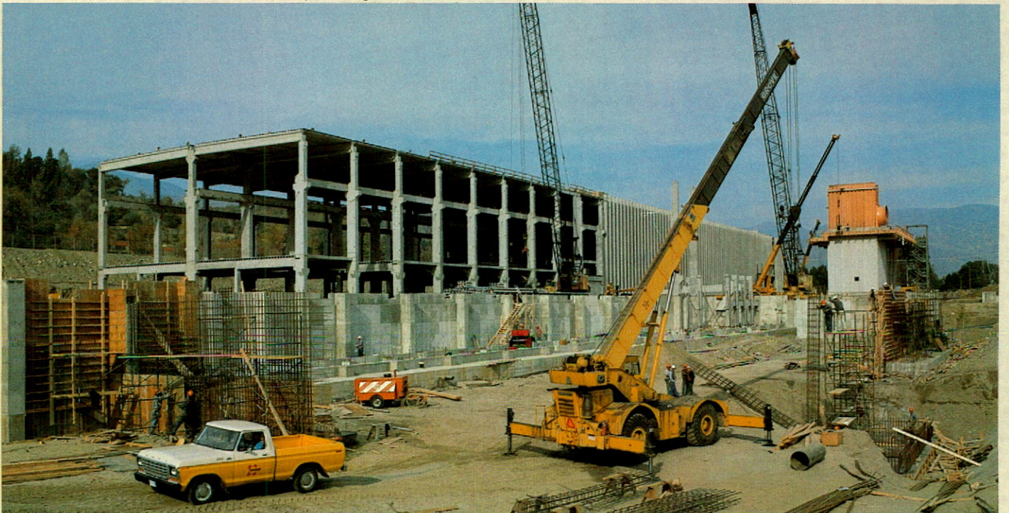
The $210 million Zinc Electrolytic and Melting Plant under construction. The largest single project in the overall modernization-expansion program at Trail, the plant will replace three existing electrolytic plants and zinc melting and casting operations.
