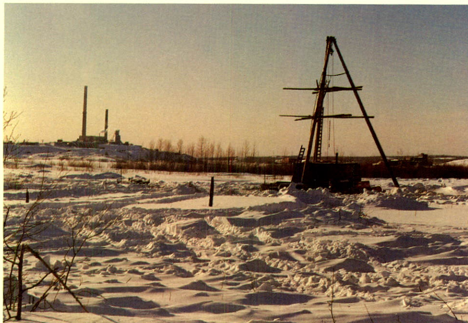
Diamond drill set-up on the Delbridge/Kerralda project, with the Noranda Horne smelter shown in background.
