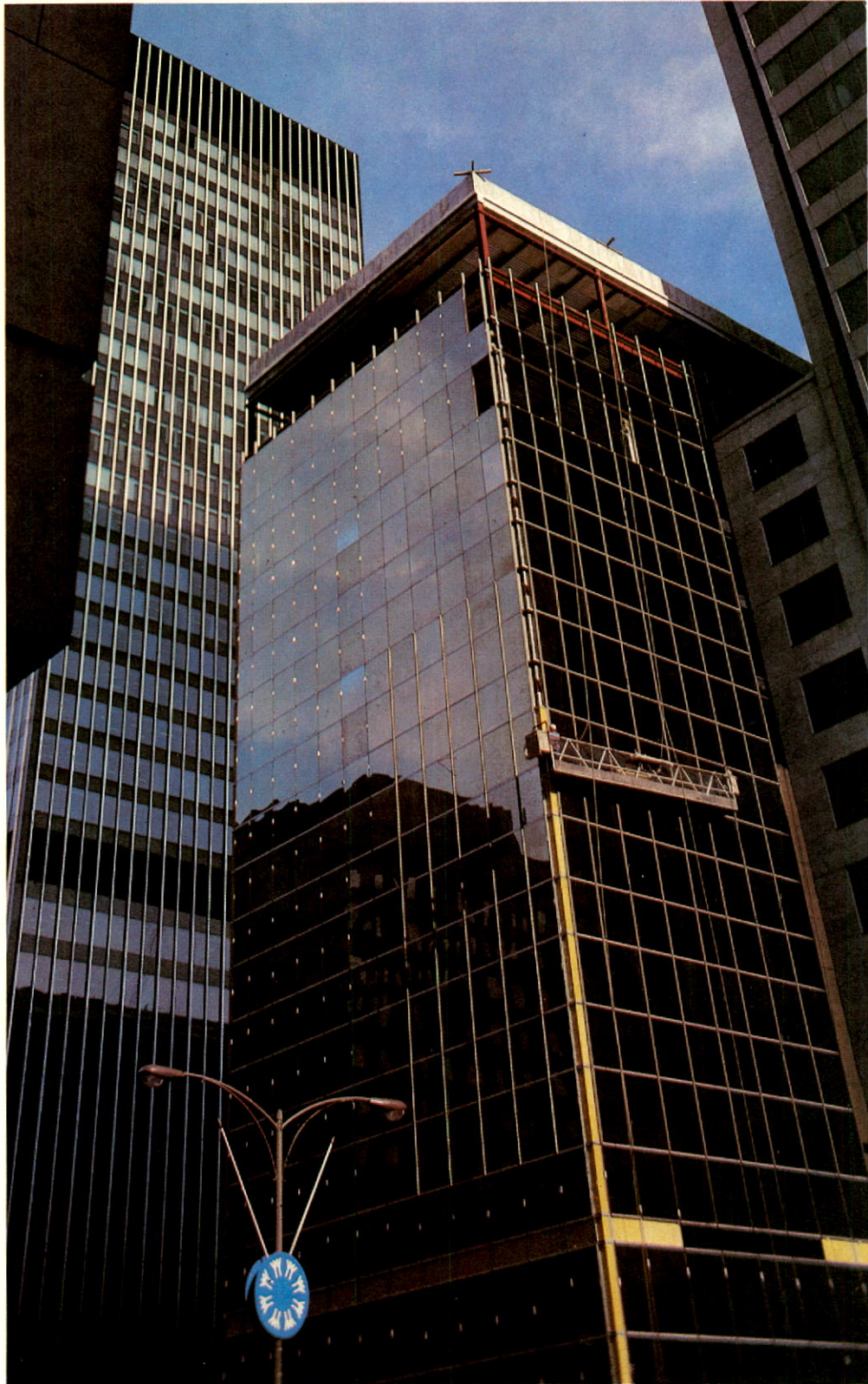
General Trust Building under construction in Montreal. A joint venture of CN's Real-Estate Division and Prenor Group.
