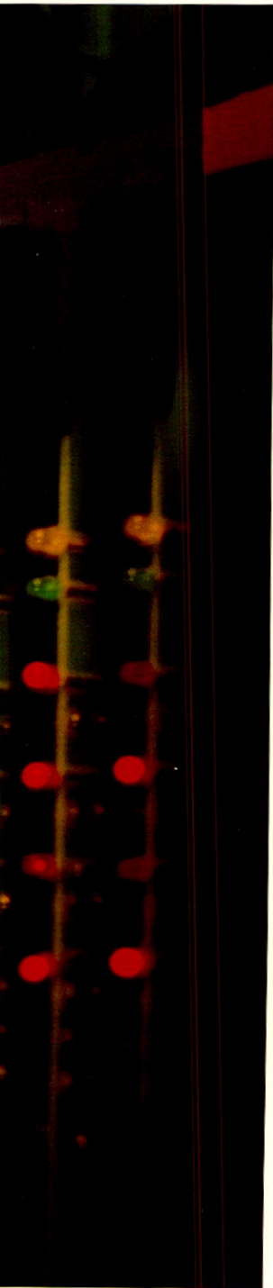
Switching centre: A technician (above) checks complex circuits at CN Communications headquarters in Toronto. The Company's sophisticated nation-wide network is carefully and constantly monitored here.
