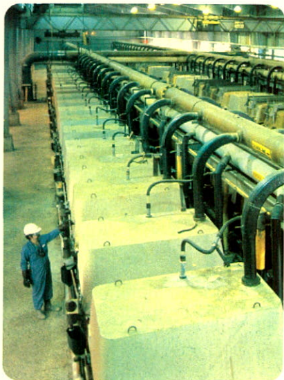
Chlorine cells at North Vancouver plant.
