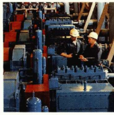
Weyburn Unit waterflood plant in Saskatchewan enhances oil recovery.
