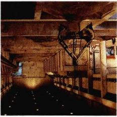
Storage bins in new feed plant for Cominco lead smelter at Trail.
