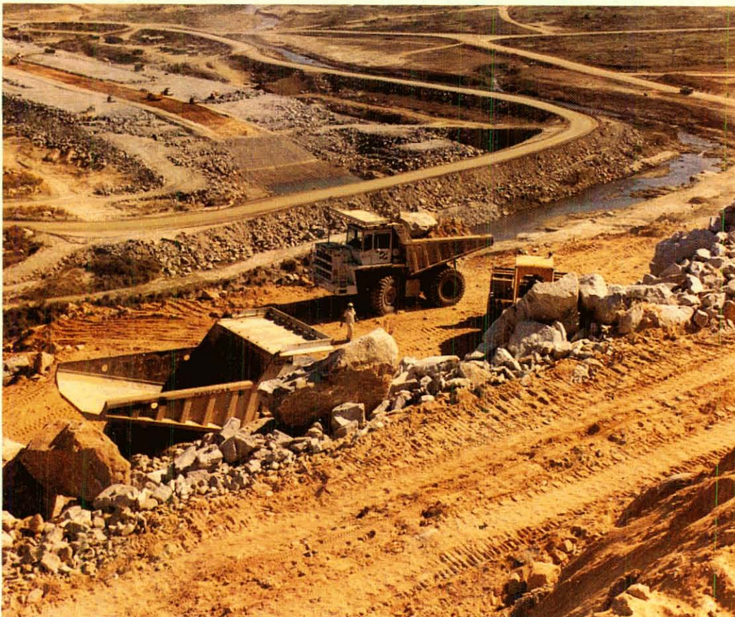
Construction of a 1000 m long by 40 m high rockfill dam, part of the Maduru Oya Irrigation project in Sri Lanka presently being carried out in joint venture.
