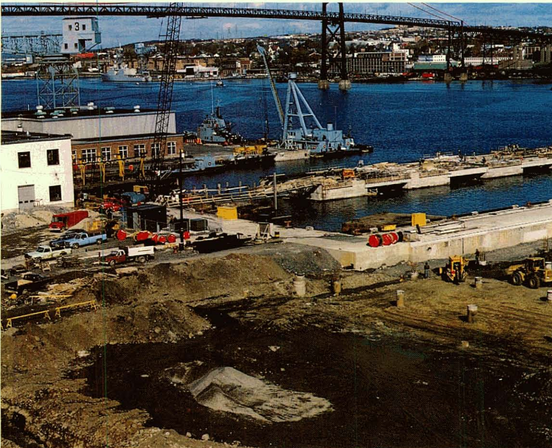
520 m long, deep-water wharf consisting of 14 concrete caissons under construction for the Ship Repair Unit (Atlantic), Halifax, Nova Scotia.
