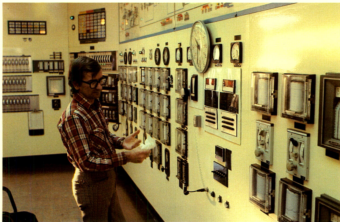
The heart and brains of the processing plant are embodied in the Rainbow plant control room
