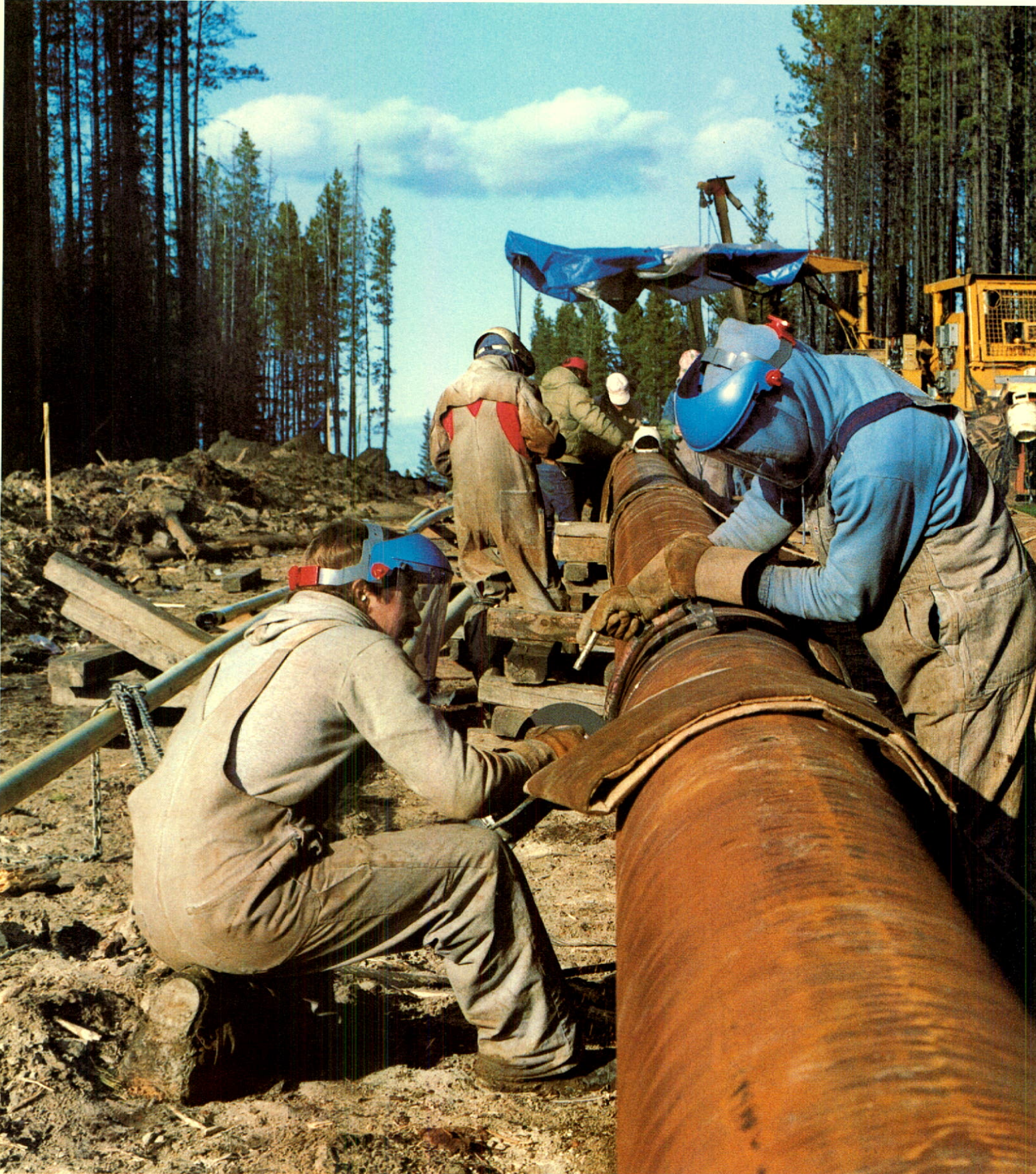
Welders join sections of the 219.1 millimetre pipe for the Hanlan/Blackstone sour gas pipeline.
