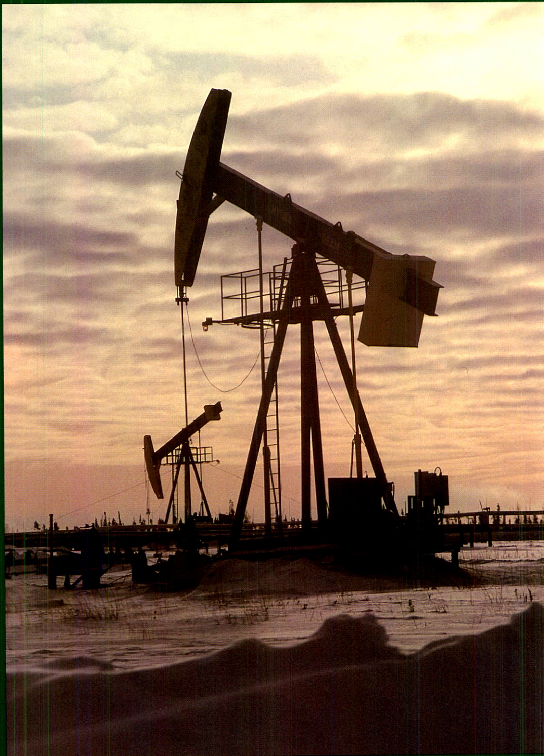
Pumping units are used to lift heavy oil to the surface at Canterra's in situ Athabasca pilot, north of Fort McMurray. Production at the pilot increased in 1984 by 68 per cent over the previous year.
