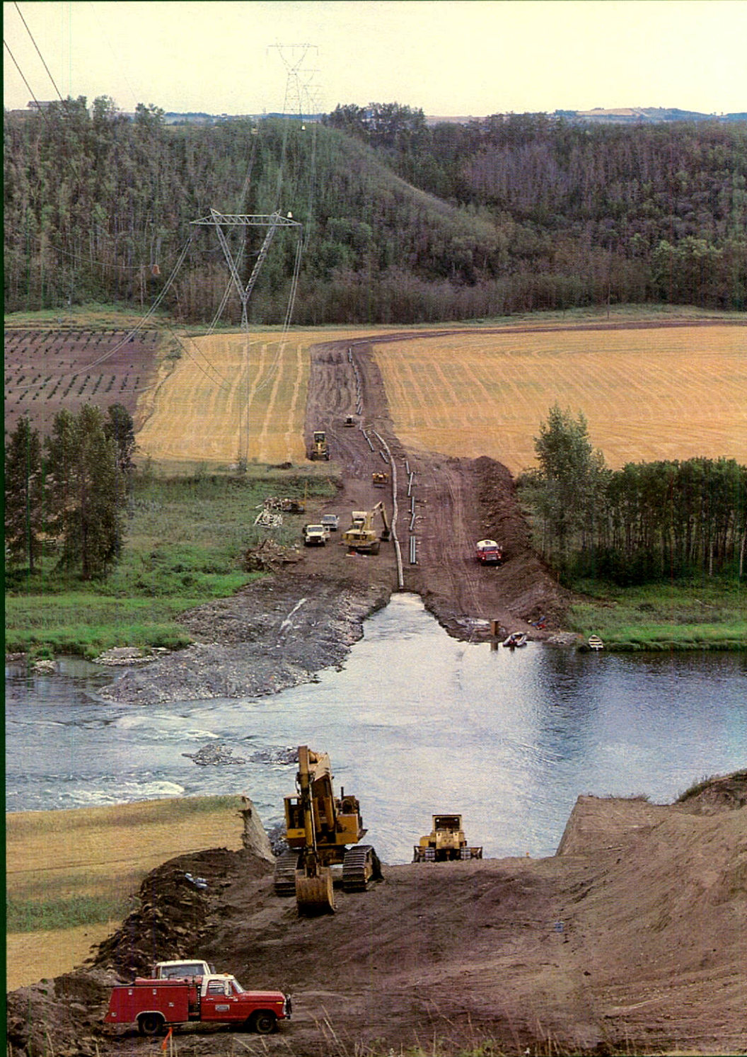
An extension line to tie in reserves near Okotoks created particular environmental challenges when the line crossed the Bow River, one of the best trout streams in North America. Precautionary measures taken to preserve the area included precise timing of the line crossing to protect fish.
