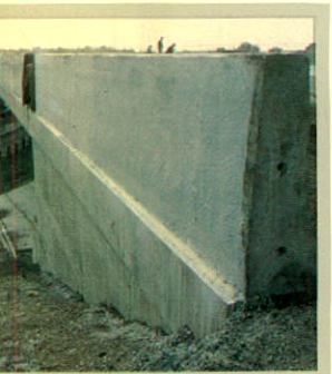
Dufferin Concrete Products continues to supply large quantities of ready mixed concrete in the construction of Highways 401 & 403 interchange in Toronto's West end.
