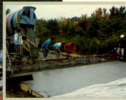
A concrete road pave-in at Belchertown, Mass. was done in cooperation with the Portland Cement Association as a demonstration of the simplicity and economy of using unreinforced concrete paving for local streets and parking lots.
