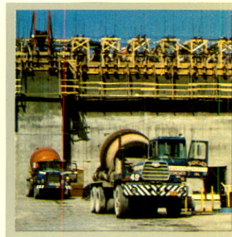
The erection of a 138 foot high bulk flour storage facility at Hudson, N.Y. utilizing the slipform concrete construction method. Cement supplied by I.C.C.
