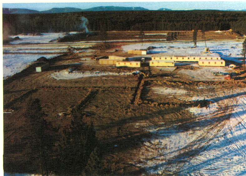
Initial construction at the Gulf-UBR $20 million gas processing plant scheduled to go on stream in November, 1970. UBR holds a 20% interest in this project.
