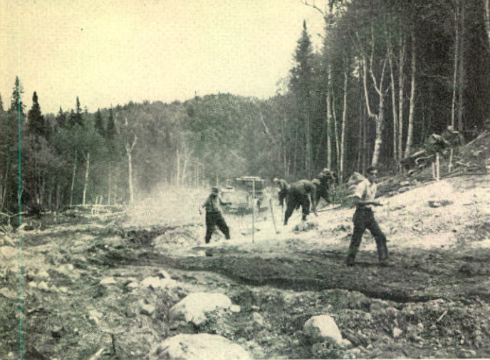
Preparing to blast a rocky obstruction during the building of the 7-mile road to the dam site.
