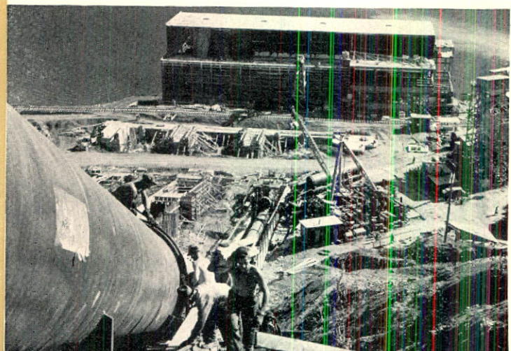
Looking down a penstock towards the power house of the Bridge River development in British Columbia.
