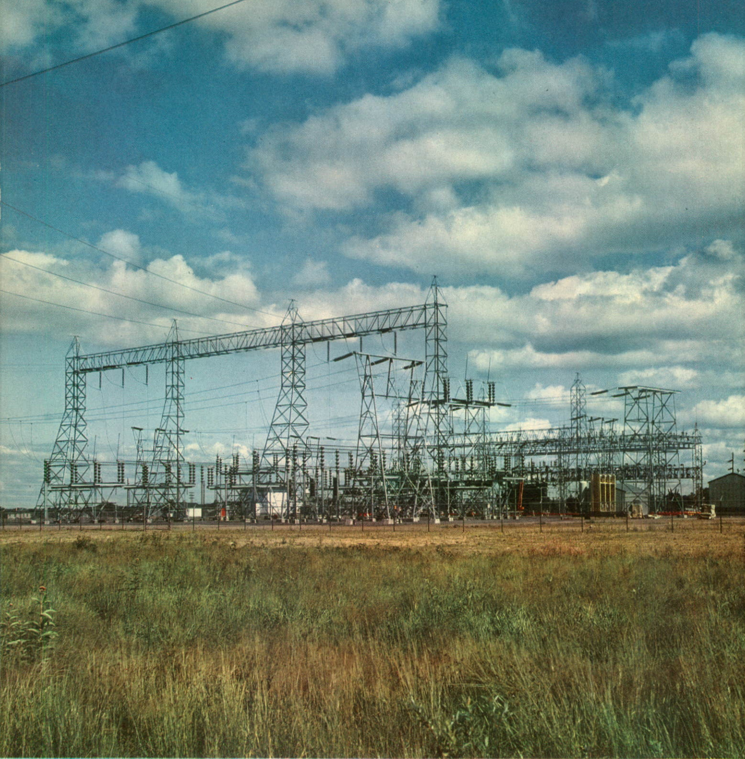
Construction of the Chaudière terminal station, shown above, which was completed in 1956, is part of a long-term programme of strengthening the Company's transmission network serving areas south of the St. Lawrence River.
