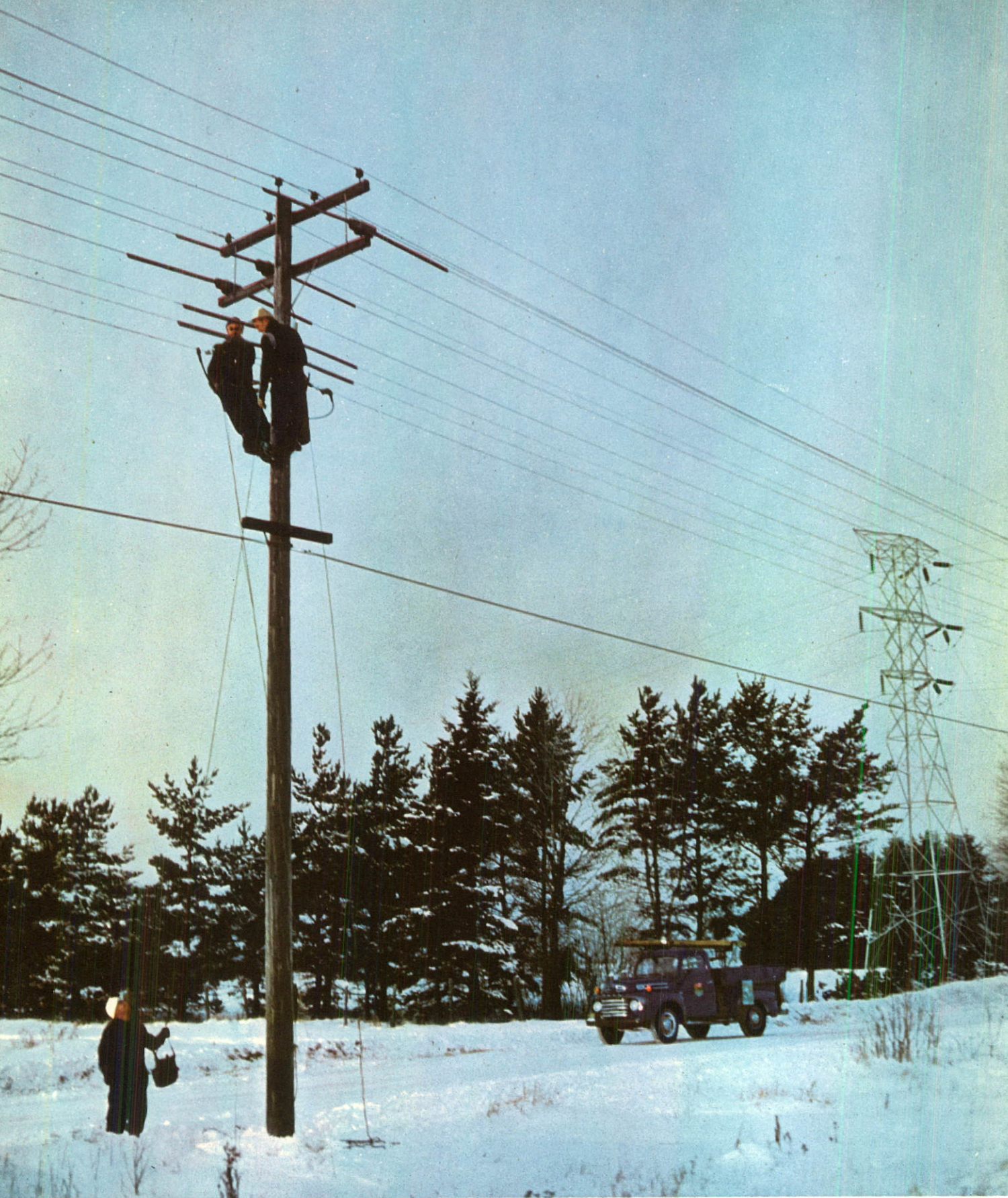
Shawinigan line crews may be called upon at any hour of the day or night and in all kinds of weather. Here a line crew is working in sub-zero weather on a distribution circuit near Shawinigan Falls.
