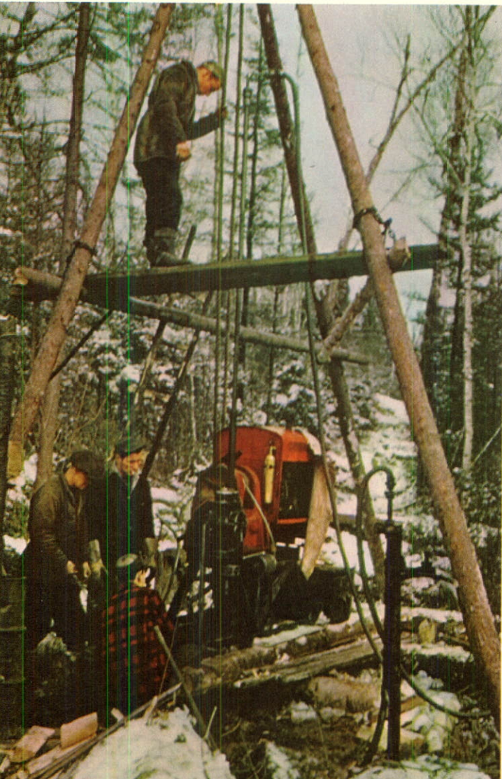
A diamond-drill crew on a survey of the Upper St. Maurice River power sites.
