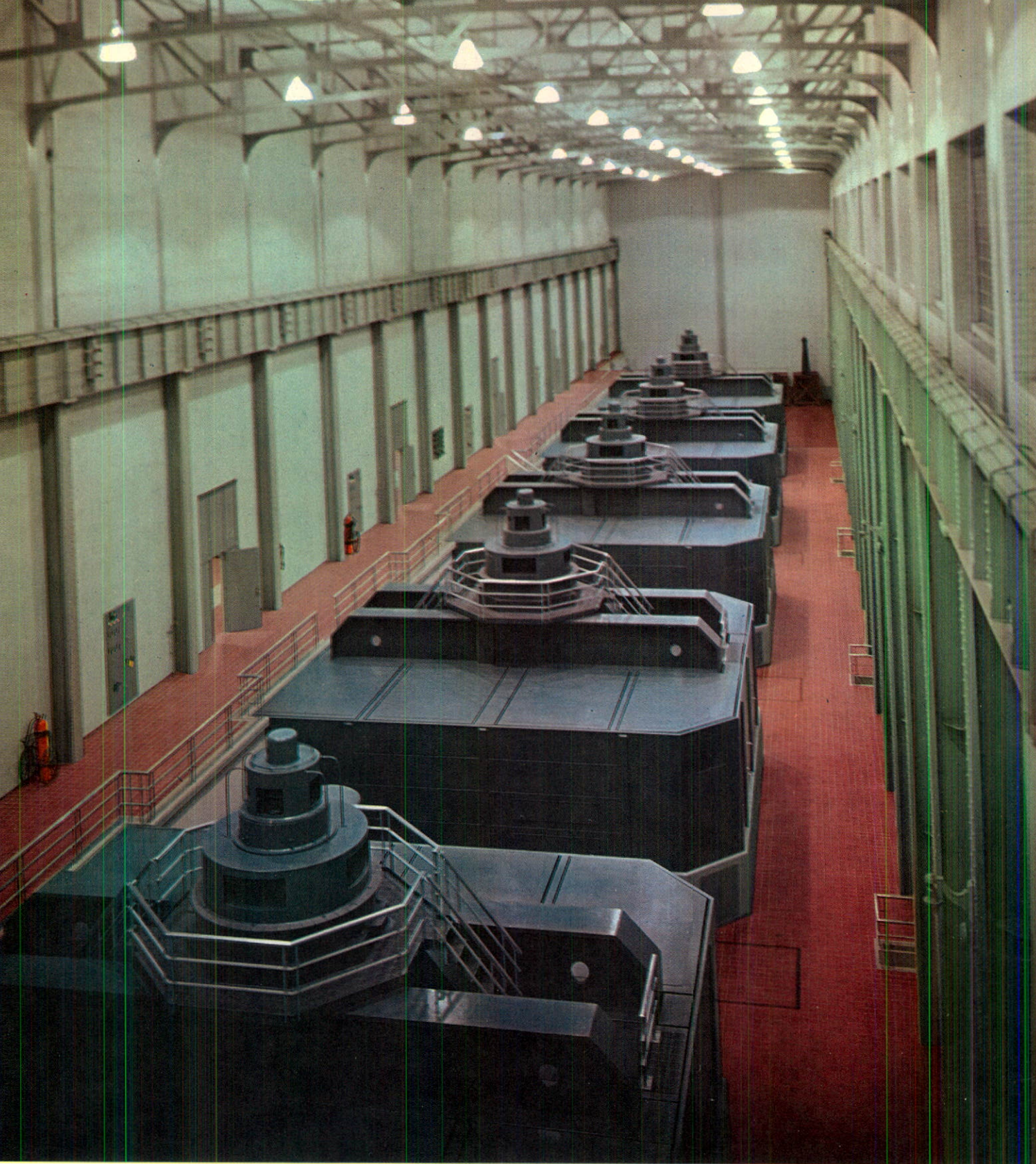
The generator room at the 325,000 horsepower Trenché development.
