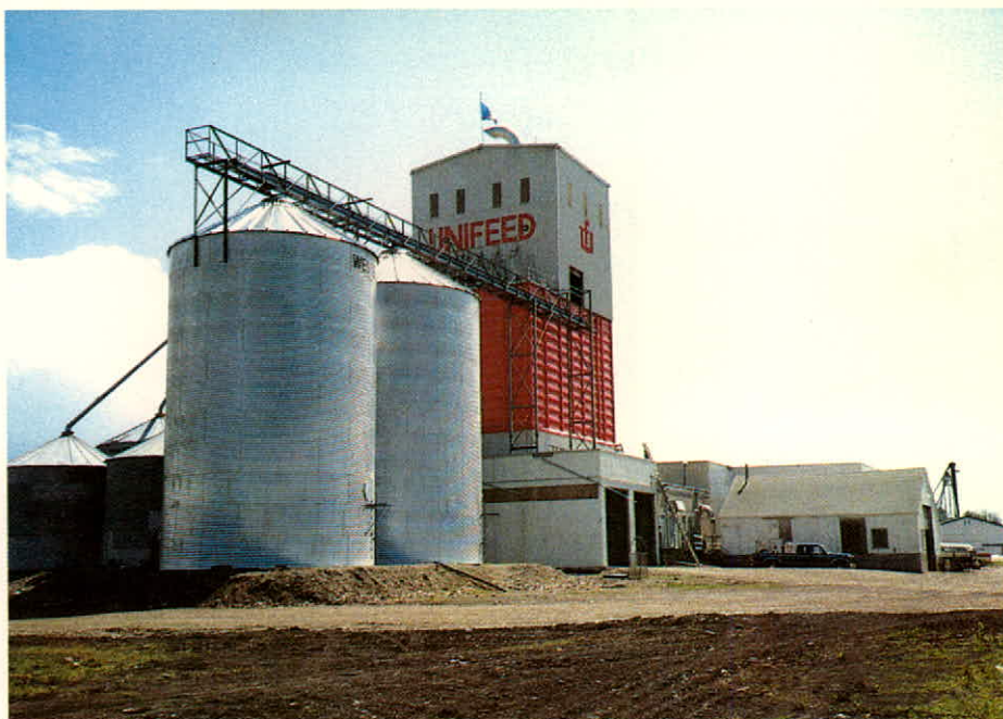
Two 20,000-bushel steel grain bins were erected at the Olds, Alta. Unifeed plant.
