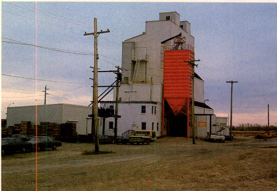
At the Midnapore, Alta. Unifeed plant, a new receiving leg was installed, as well as a cluster of steel load-out bins.
