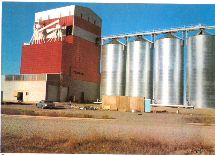
Construction of the first phase of the new feed mill at Lethbridge, Alberta is completed. The second phase, including grinding, pelleting and bagging facilities plus the warehouse and office, has started.
