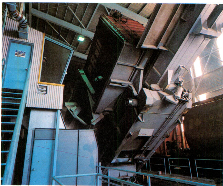
Both boxcars, by a mechanical dumper, and hopper cars can be unloaded simultaneously. The hopper cars are unloaded into a new discharge pit, installed as part of the Vancouver terminal renovation.
