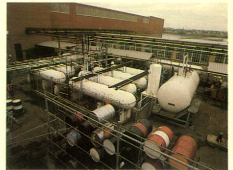
Bulk propellant storage facilities
