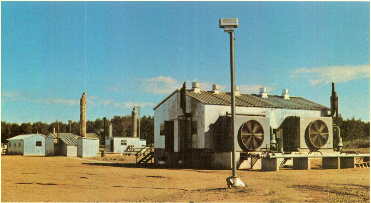
Provident natural gas compressor facility near Warwick, Alberta.
