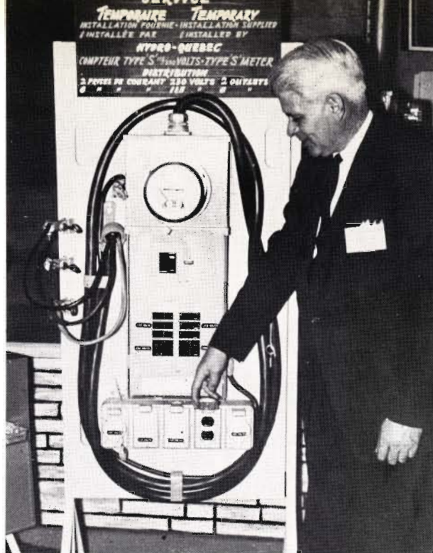
Temporary connection panel to facilitate and accelerate the supply of service to builders and contractors.
