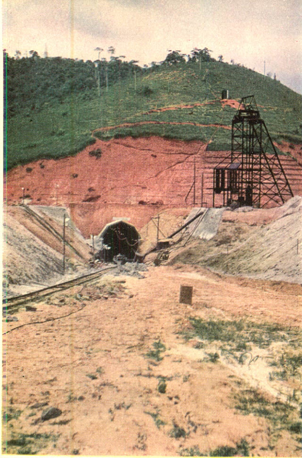
EXCAVATION FOR VIGÁRIO TUN- NEL TO CARRY WATER FROM PARAÍBA RIVER TO FONTES POWER PLANT.
