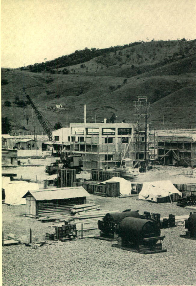
CONSTRUCTION OF APARECIDA STATION WHERE A 50,000 KW. FREQUENCY- CHANGER IS BEING INSTALLED. .....
