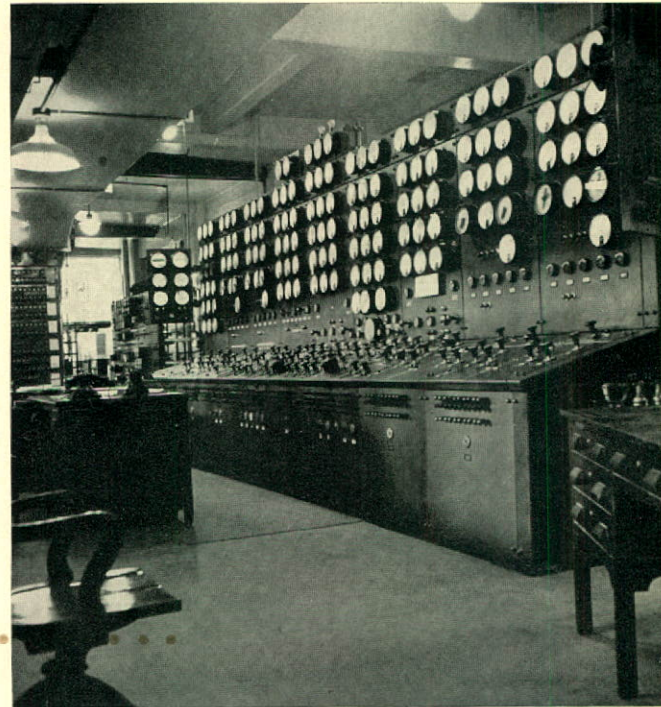
CONTROL ROOM AT SERRA DO CUBATÃO POWER PLANT. .....
