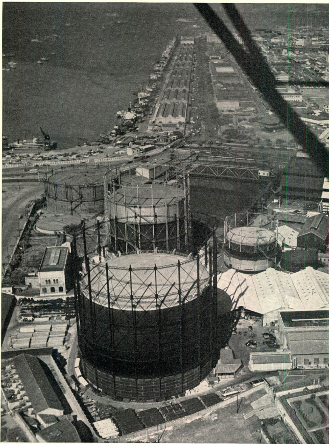
RIO GAS WORKS FROM THE AIR SHOWING, LEFT CENTRE, NEW 85,000 CUBIC METER GASHOLDER UNDER CONSTRUCTION.
