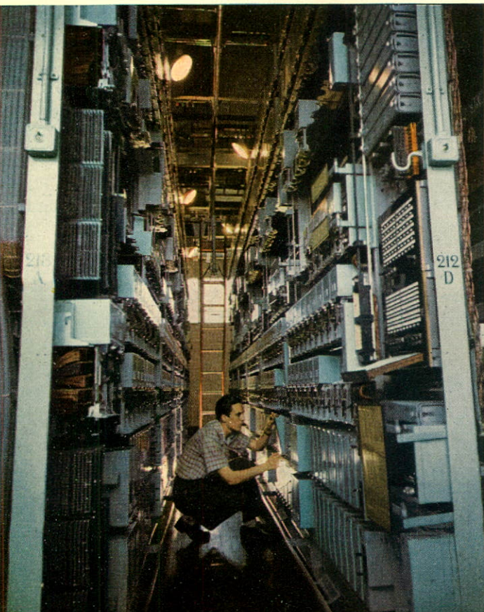
THE NEW AUTOMATIC TELEPHONE EXCHANGE INSTALLED IN SÃO PAULO IN 1950.
