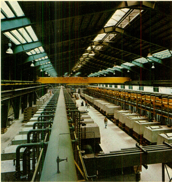
ICI-Solvay diaphragm cells were installed in the new cell room at Bécancour.
