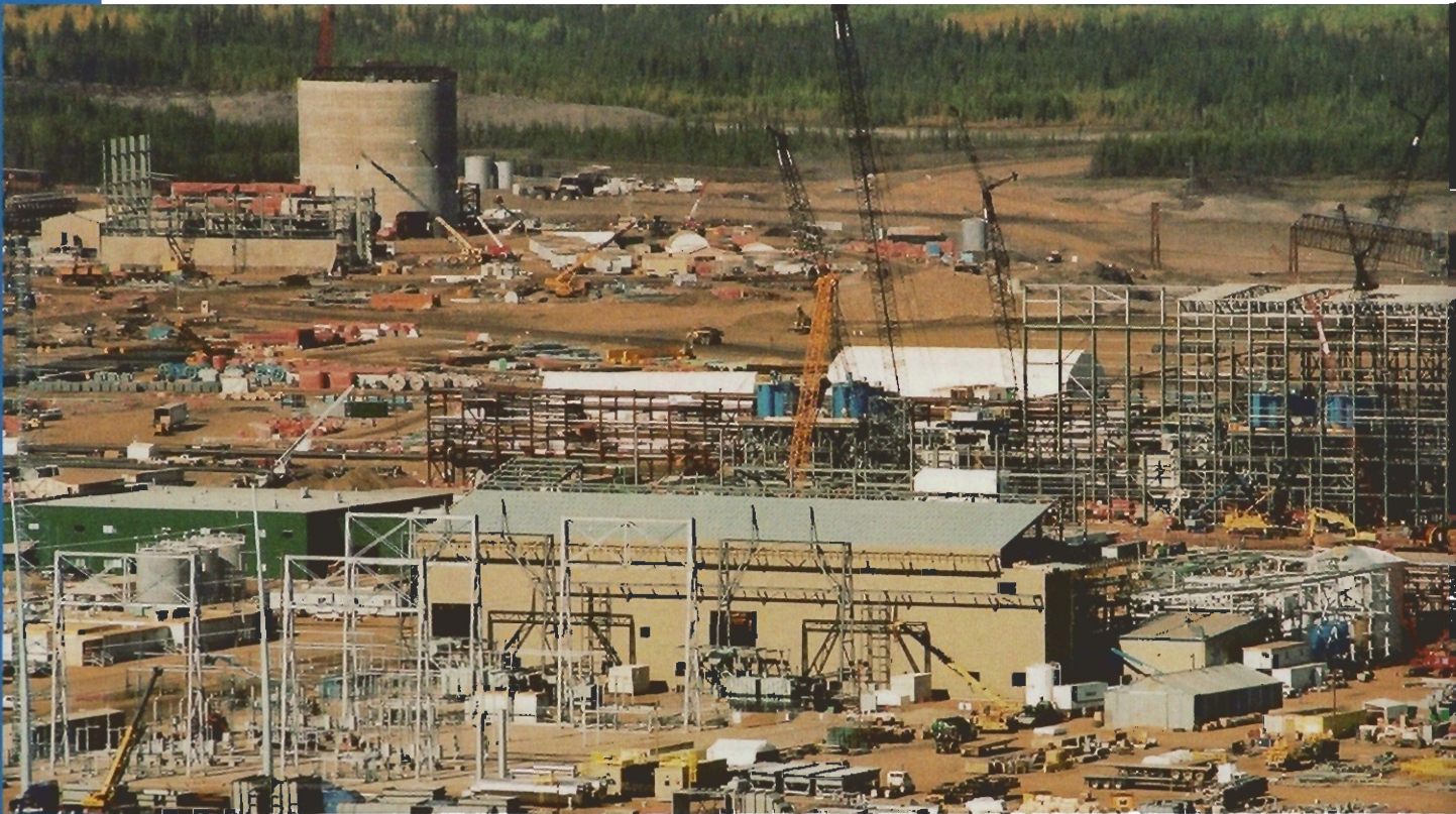
Muskeg River cogeneration plant, near Fort McMurray, Alberta
