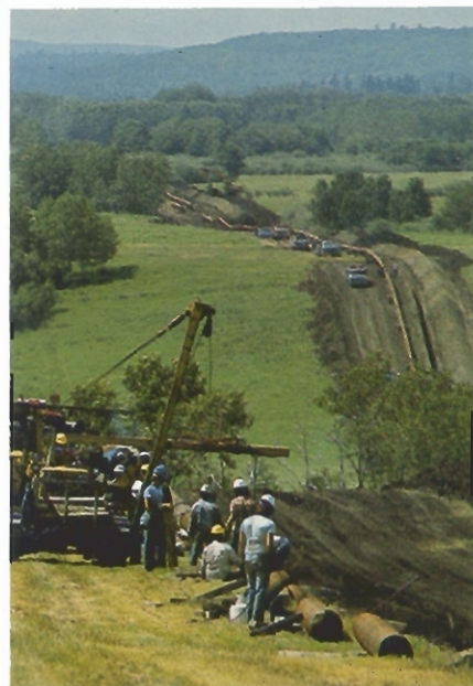
Above: Crews lay transmission pipeline, one of the projects totalling $37 million during the year to meet growing service obligations of Canadian Utilities Limited. Left, below: A natural gas regulating station in Calgary, typical of numerous installations operated to provide utility service.
