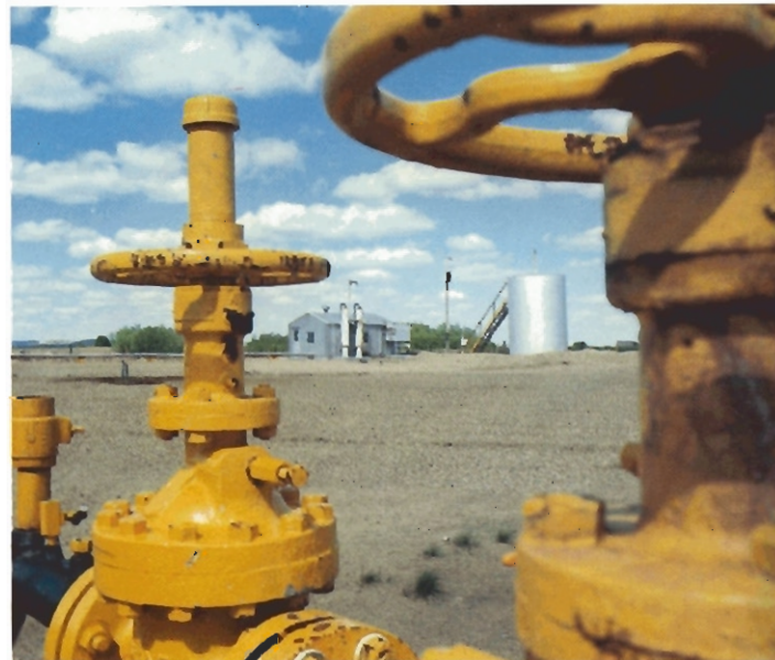
ATCO gas plant in the Province of Alberta.
