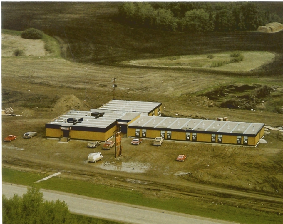
Upper left: A 300-ton crane to be barged in for Denwood Motel
