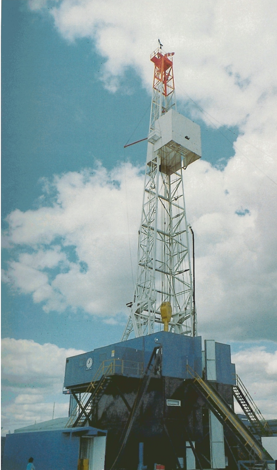
Left: The first rig, a National 80 UE, of Mustang Drilling's major expansion program on the rig up with Edmonton, Alberta
