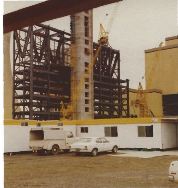
Office and washroom facilities on urban power station project 300 man camp at Luscar Ltd. coal mine site, Coal Valley, Alberta
