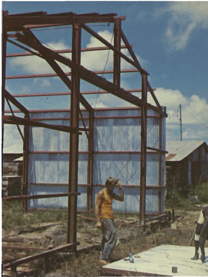
Westinghouse repair and maintenance centre — Saudi Arabia
