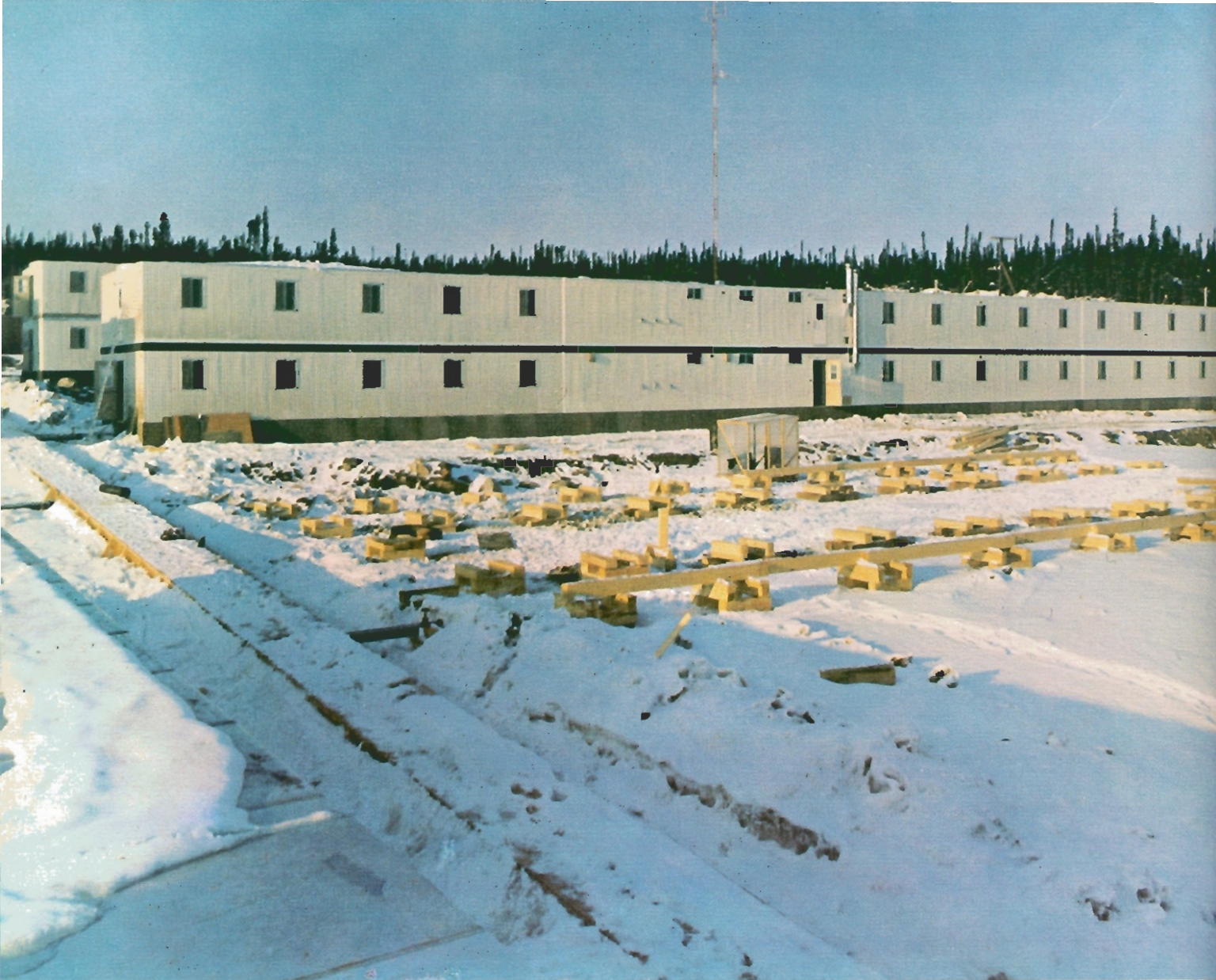
2-story barrack blocks housing Quebec Cartier workmen at their giant new iron ore mine in Northern Quebec.
