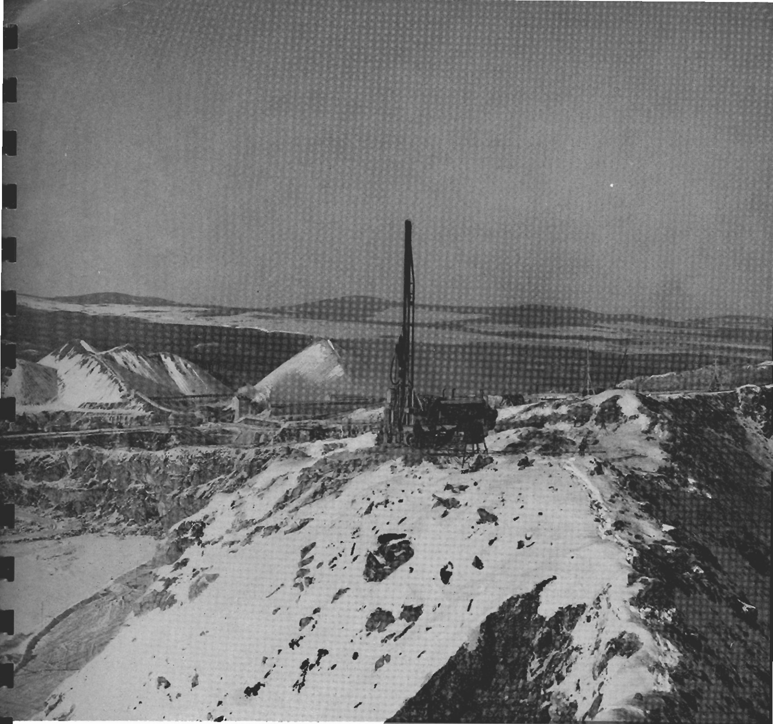
A New Type of Self Propelled Rock Drill in Operation at British Canadian Mine.
